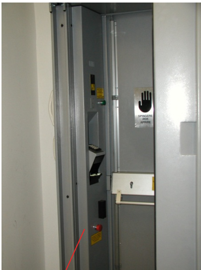
EMERGENCY PUSH BUTTON TO UNLOCK BOTH DOORS
